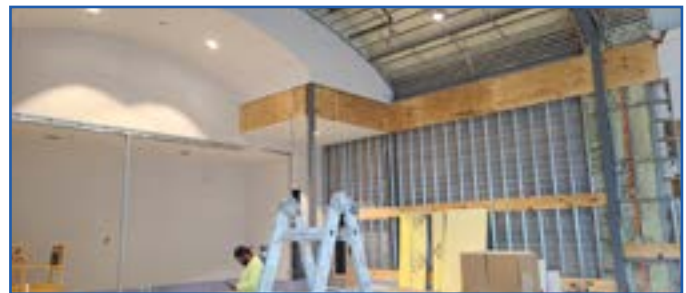
Drywalling continues in the chancel area. The left side of the picture is the back wall.
