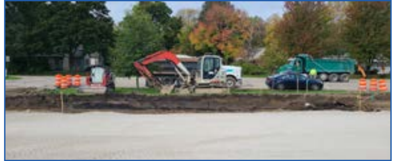
A stone base is being laid in the excavated parking lot. Facing west toward Santa Monica.
