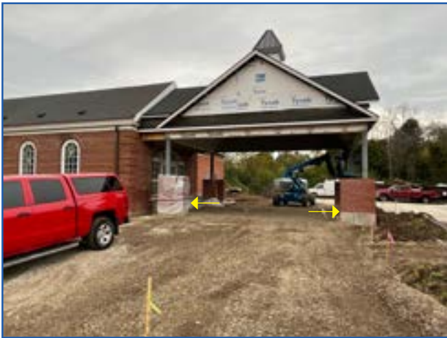
The driveway is being sloped to meet the doorway under the porte cochere. It will be as high as the yellow arrows in the picture to the left.
